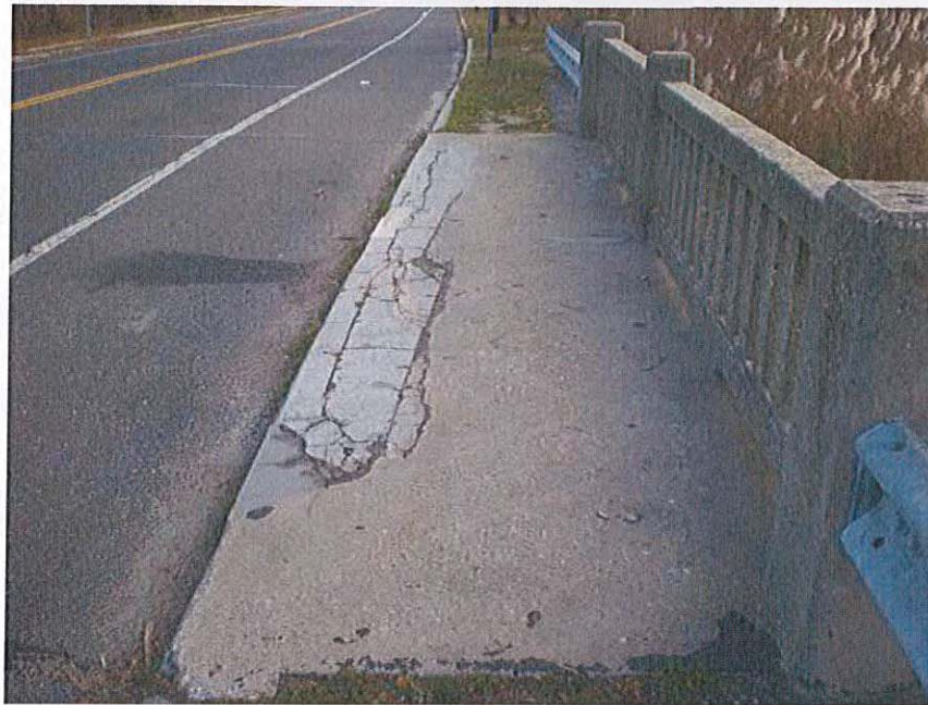
South side of bridge – looking east - cracked sidewalk
