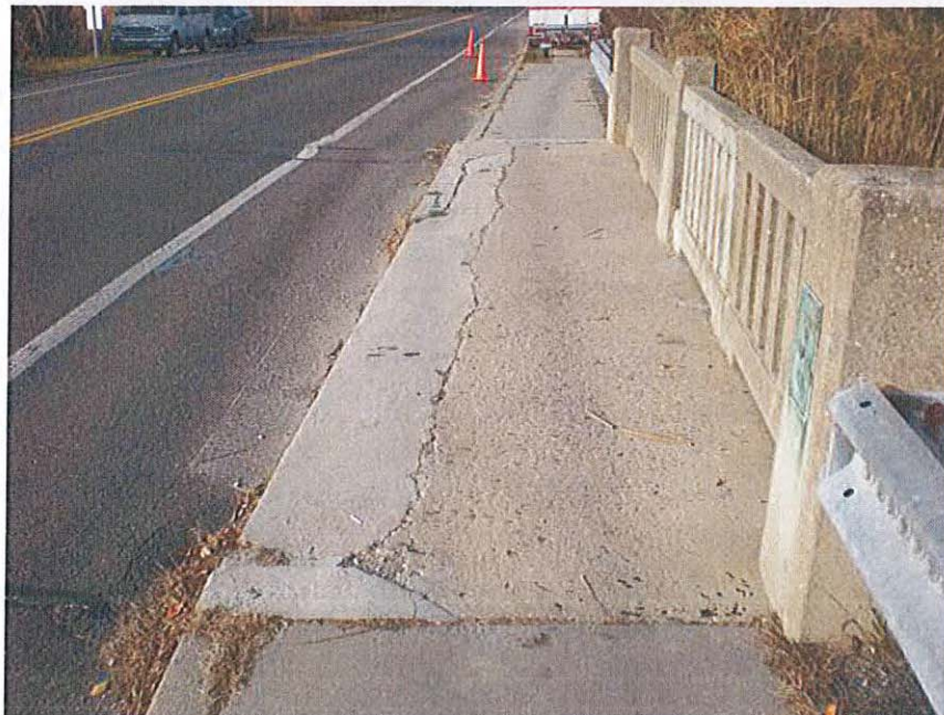
North side of bridge – looking west - cracked sidewalk
