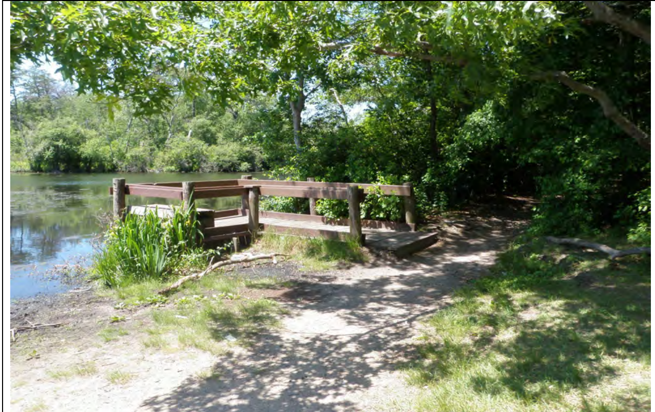
PHOTO #5: View north showing existing boardwalk structure within mitigation Area 1 which is nonfunctional.
