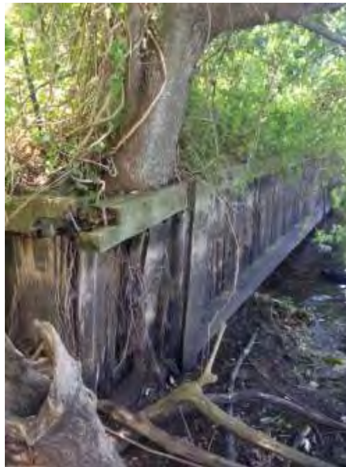
Photo 4: Abandoned Wooden Bulkhead
