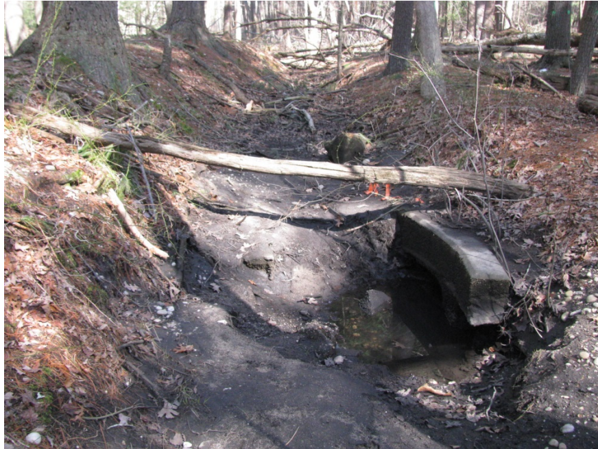
LOOKING NORTH (UPSTREAM) AT EXISTING HEADWALL SHOWING CARMANS RIVER STREAMBED (NOTE LITTLE EVIDENCE OF FLOW)
